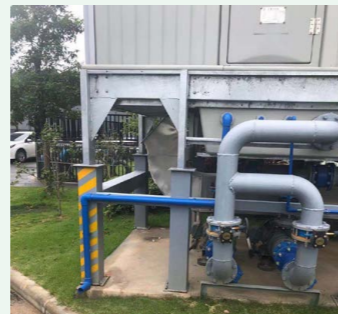
Sewage pipeline of the cooling water tower
